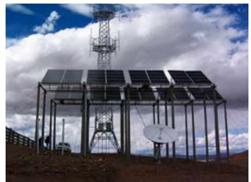
Telecommunication station in Xinjiang. System integrator: TBEA Xinjiang Sunoasis Co., Ltd.
