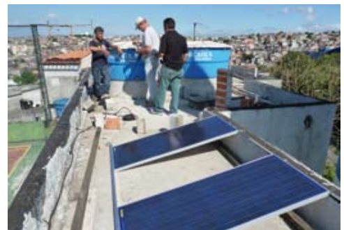
On top of the Casa do Zezinho School. Module supplier: Solara. System integrator: Preserva Solar.
