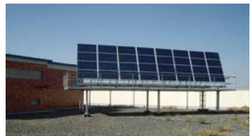
Solar gas pipeline power system in Qinghai. System integrator: TBEA Xinjiang Sunoasis Co., Ltd.
